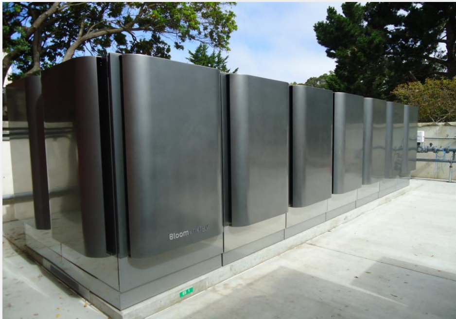
Figure 4 - 200kW Bloom Energy Server Installation
